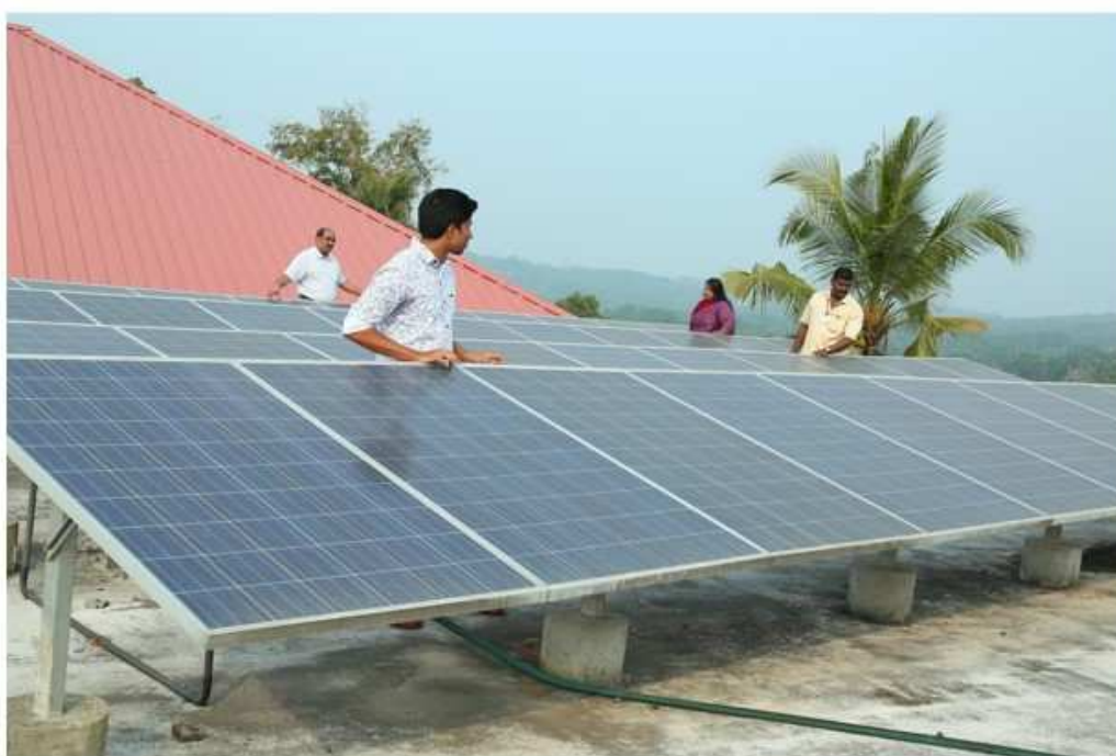
Plate V. B Students and teachers inspecting the Solar Power plants installed in Nirmala College.
